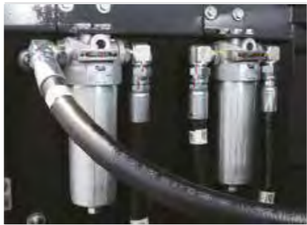
Protected hydraulic system
